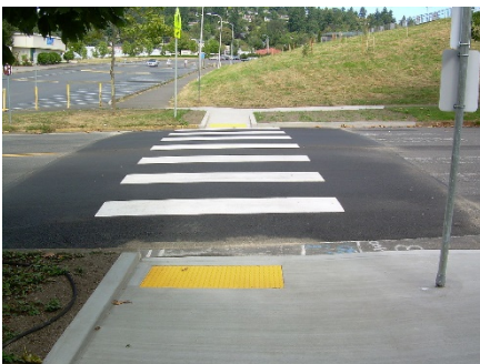
Raised Crosswalk. SOURCE: Scott Batson
